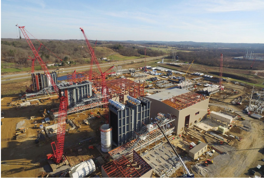
Guernsey Power Station Byesville, OH
